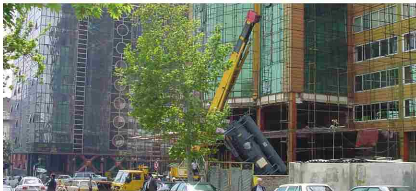
Transport to Mechanical Room
